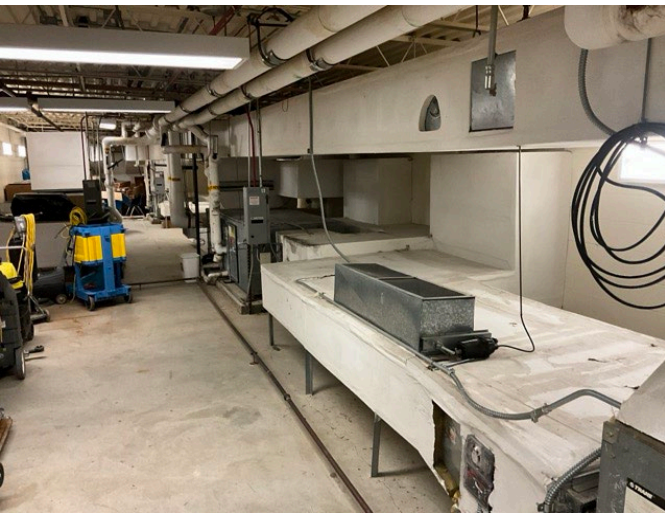
21 - SECONDARY MECHANICAL ROOM
