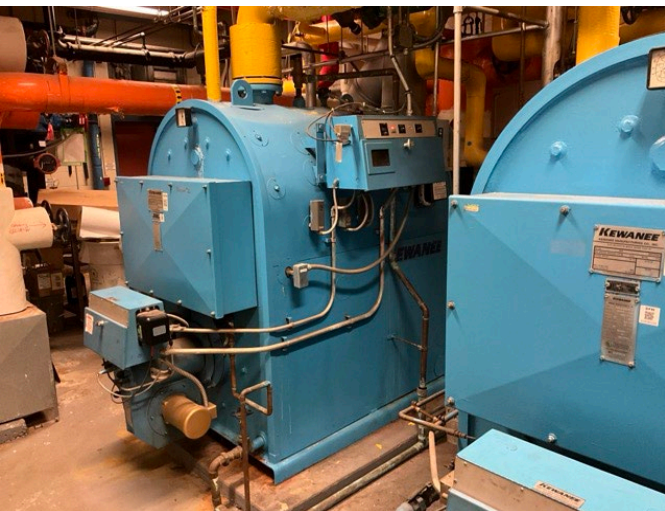
23 - MAIN MECHANICAL ROOM
