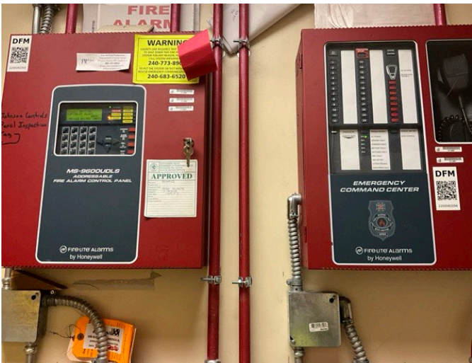
27 - FIRE ALARM PANEL
