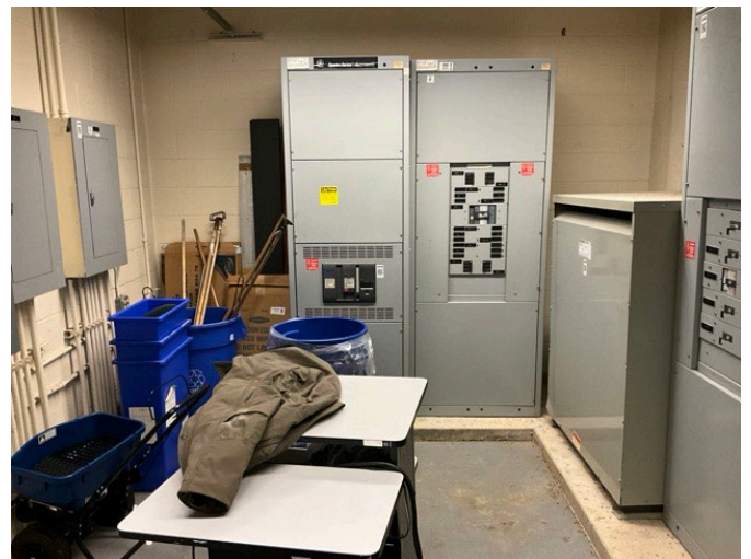
24 - MAIN ELECTRICAL ROOM
