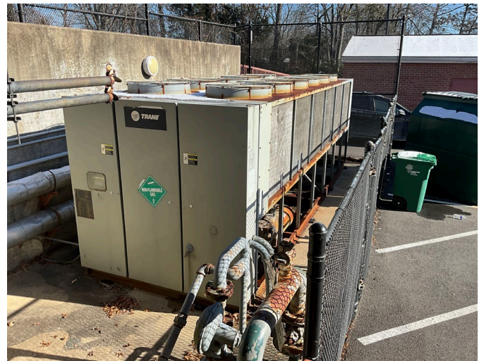
22 - CHILLERS AND PUMPS
